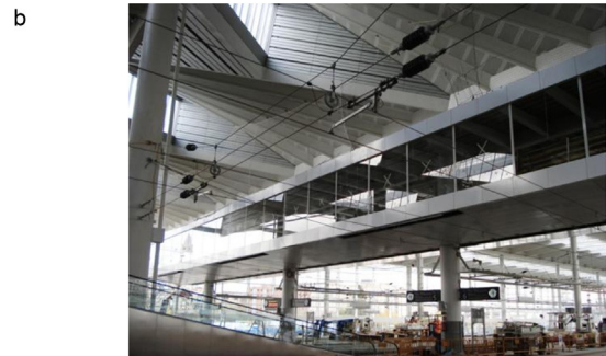
Figure 7. (a) Méndez Álvaro footbridge, plan view. (b) Méndez Álvaro footbridge, photograph taken during construction.
