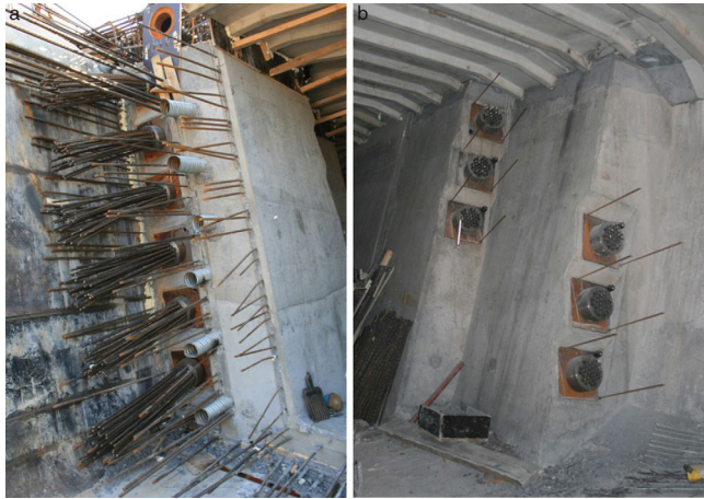
Figure 28. Continuity tendon anchorages and crosslinked wires and active anchorages at cantilever front; passive steel anchorages.
