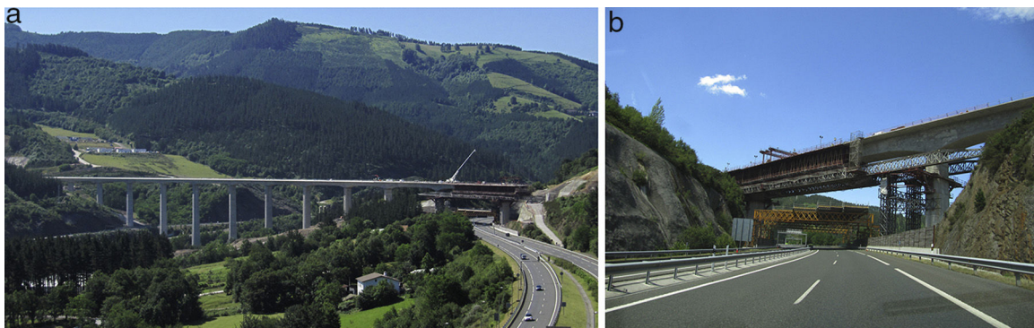
Figure 30. MSS on the 80 m span over motorway AP-1, which presently holds the record in Spain for high-speed rail viaducts built with this system.
