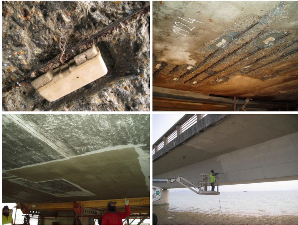
Figure 6. Details of the repairing procedure (sacrifice anodes, application of mortar patches and final painting).
