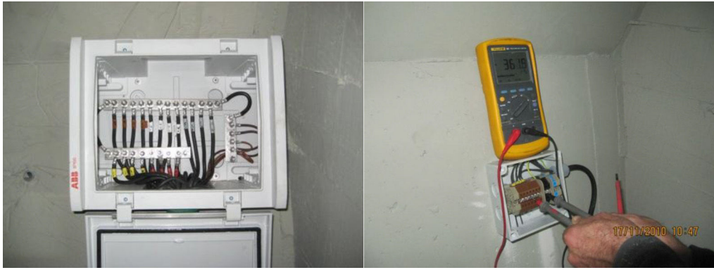
Figure 9. Detail of a connection box and the procedure of measurement of the voltage.
