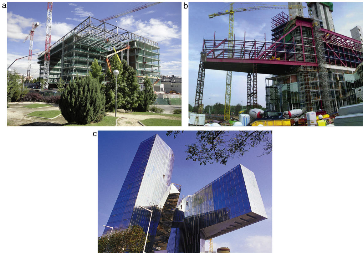
Figure 10. Building and roof of the Data Processing Centre in the execution stage (above), Gas Natural headquarters building in Barcelona (below).
