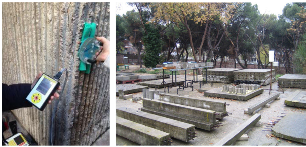
Figure 8. Left the corrosion rate meter in a column with rough finishing. Right: exposure site and the garden of the IETcc to study the effect of the climate into the corrosion of several concrete elements.
